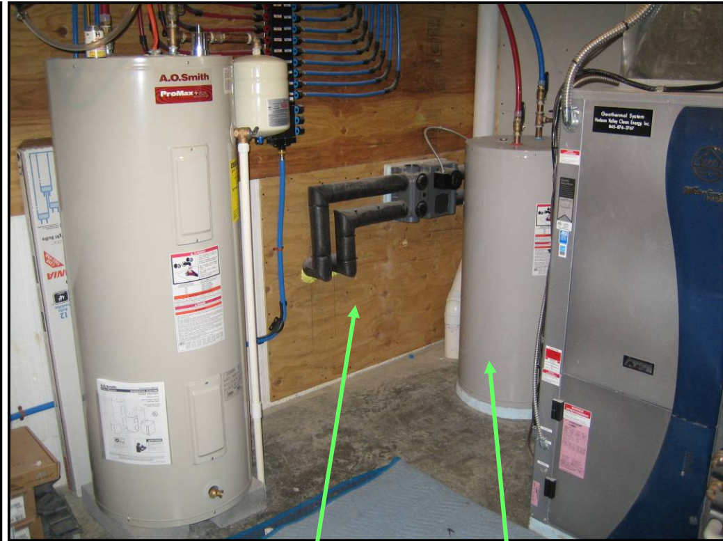
Pre-tempered water tank
